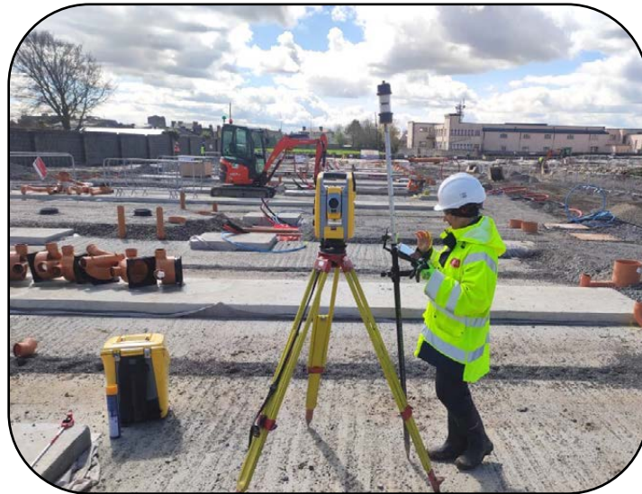
• Tania at work in Thurles, Co. Tipperary, on the site of modular housing for fellow Ukrainian refugees.
